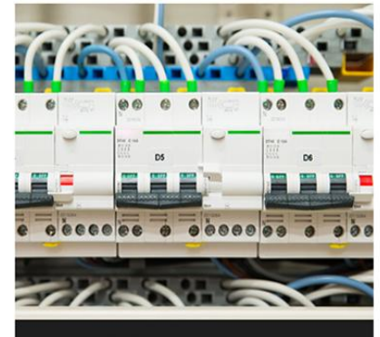
CONFIDENTIAL GLOBAL MANUFACTURER - CONTROLS RETROFIT
