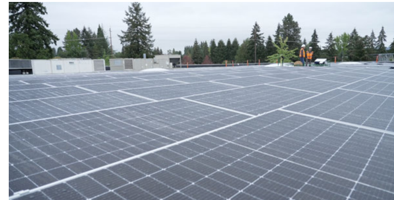
Dynalectric Oregon completed this new solar installation for a manufacturing facility, helping the client achieve their sustainability goals and minimize operating costs.
