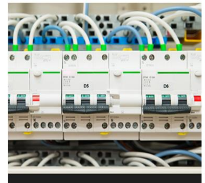
CONFIDENTIAL GLOBAL MANUFACTURER - CONTROLS RETROFIT
