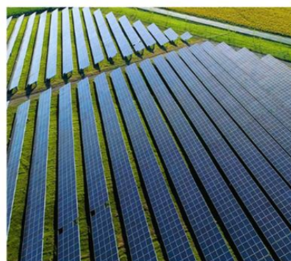
FREEMONT COMMUNITY SCHOOLS - SOLAR FARM
